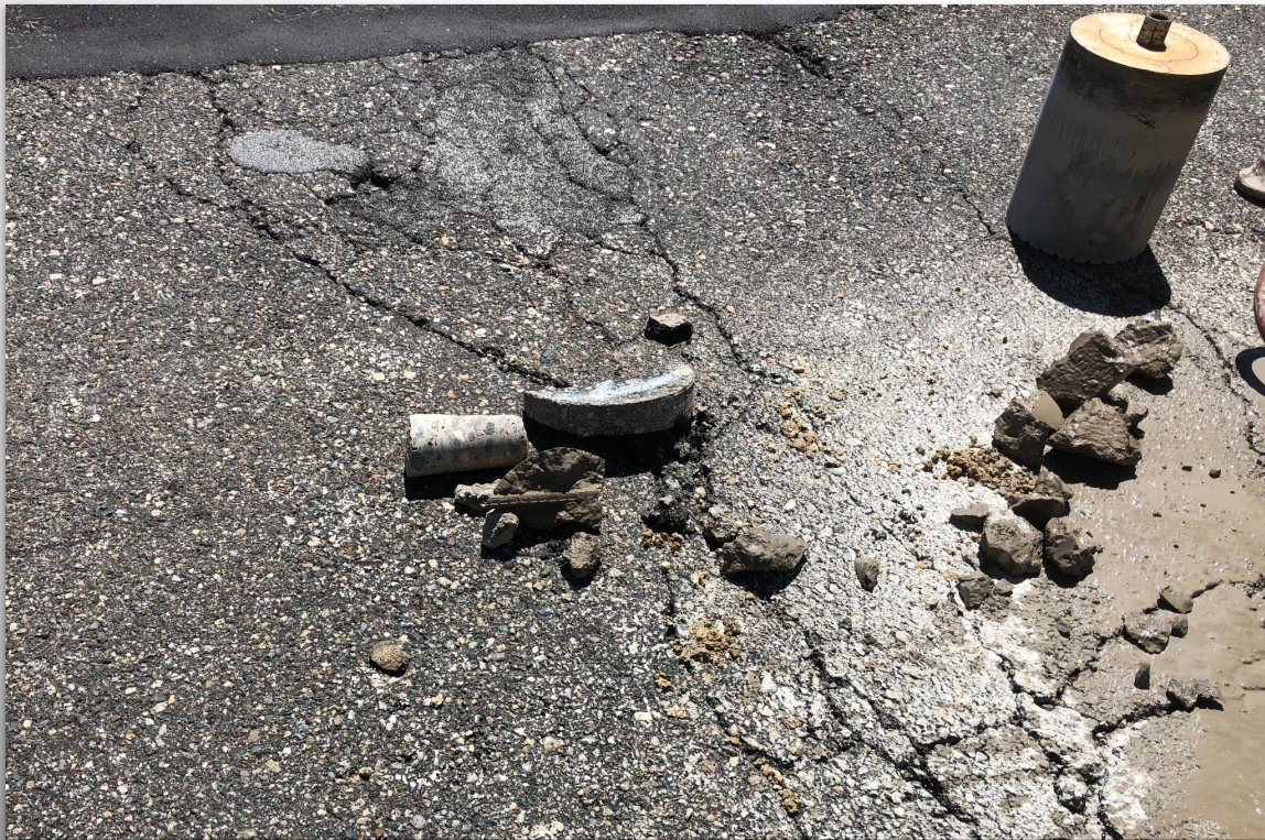
Pavement Core in failed pavement area
