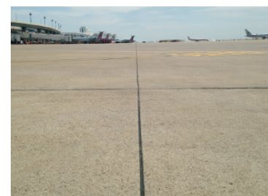
40-year-old Preformed Compression Seal at DFW Airport.
