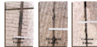
Figure 3. Failure modes of joint seal materials at the Mesa SPS-4 site.
