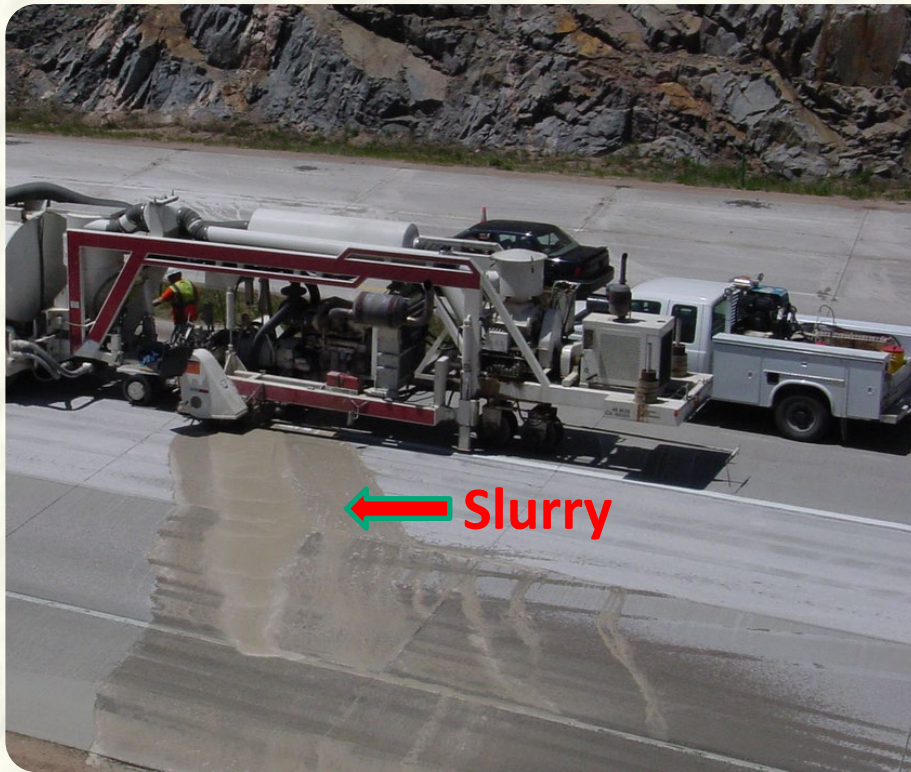
Slurry Recovery Failure
