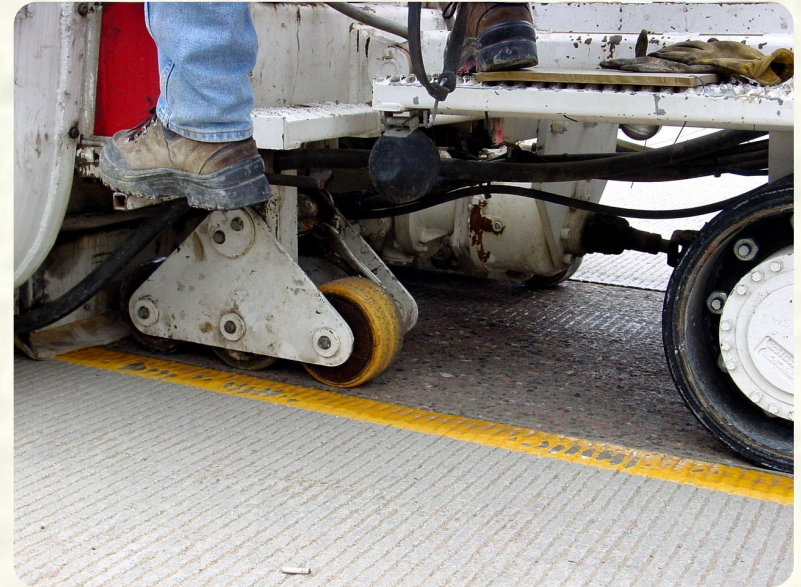
Proper Slurry Recovery System
